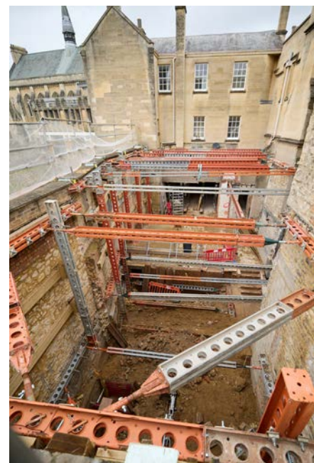
The kitchen space while underpinning work was underway in the spring—the SCR rooms and Hall are on the right and the Balliol wall on the left
